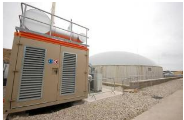
Image 5; SGN plant and anaerobic digesters at Poundbury
