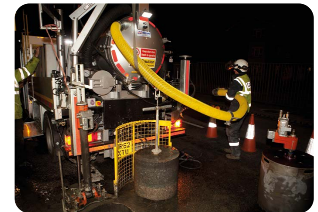
Core and Vac allows us to carry work through small keyhole excavations, vastly reducing the scale of our work and traffic management required.
