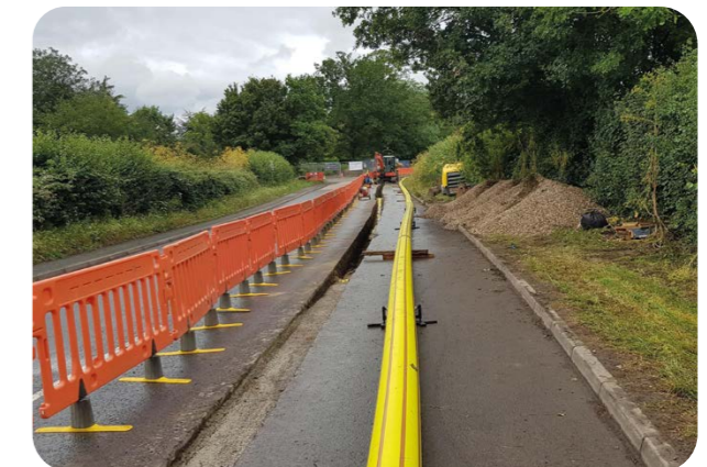
We’re replacing old metal mains with PE pipe – the key material we procure in terms of spend.
