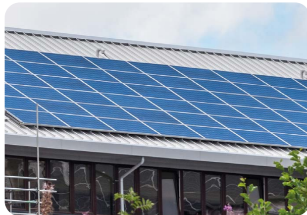
We're aiming to have direct feed solar panels on all of our occupied sites.
