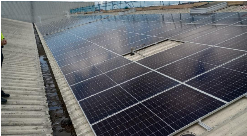
PV cells on roof
