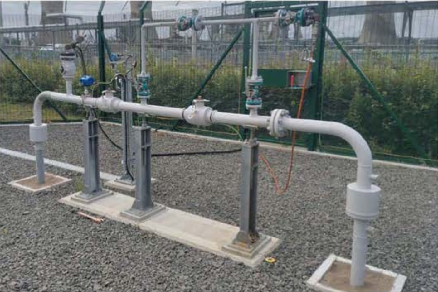
Figure 5: Bo'ness Road compound – hydrogen isolation point.
