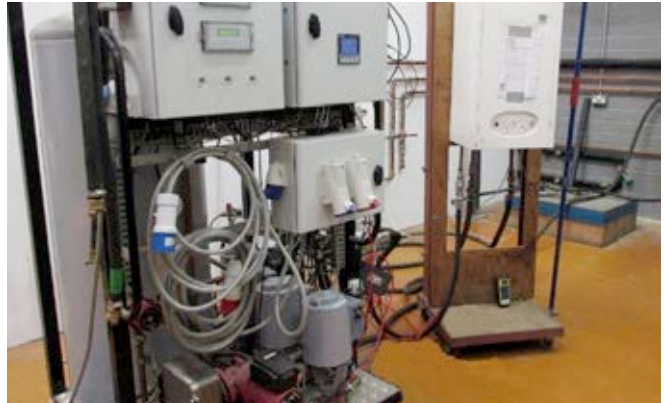
Boiler in laboratory
